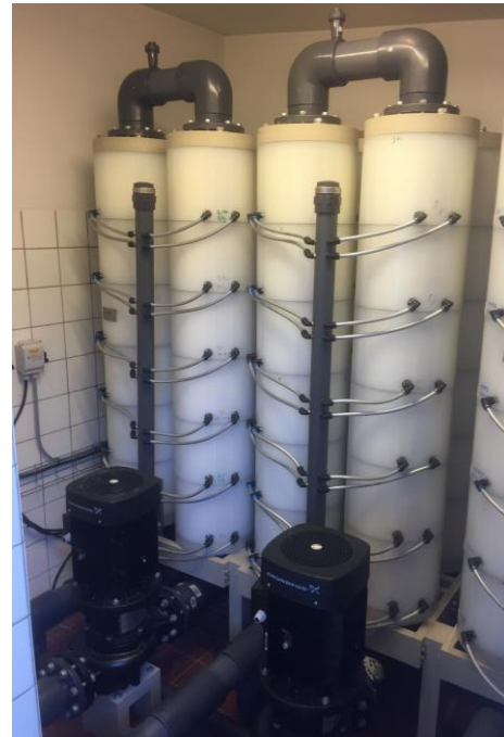
Part of a MF/UF cascade Free Flow Plate™ cross flow plant
