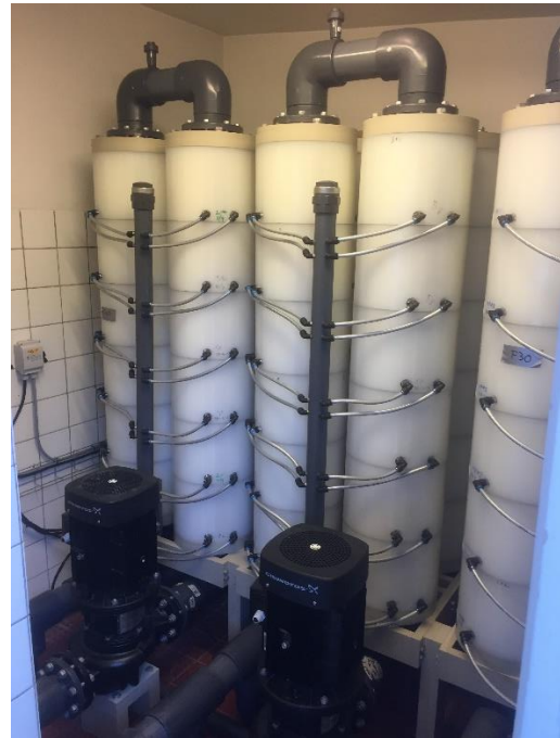
Part of a MF/UF cascade Free Flow Plate™ cross flow plant
